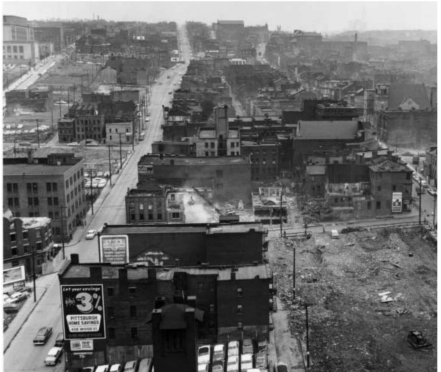
Beginning of demolition of the Lower Hill, ca. 1955. Source: Allegheny Conference on Community Development Photographs, 1892-1981, MSP 285, Library and Archives Division, Senator John Heinz History Center
